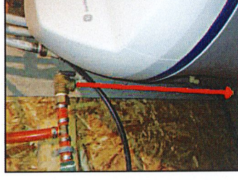
Missing TPRV extension
